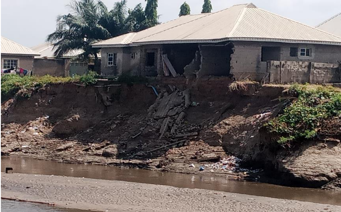
Plate 1: Poor Proximity to River Channel (Source: Author’s Fieldwork, 2025)
